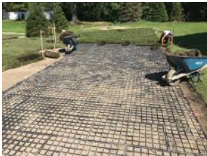
Installation of GEOBLOCK® pavers over prepared engineered base. Infilling the pavers with topsoil.
